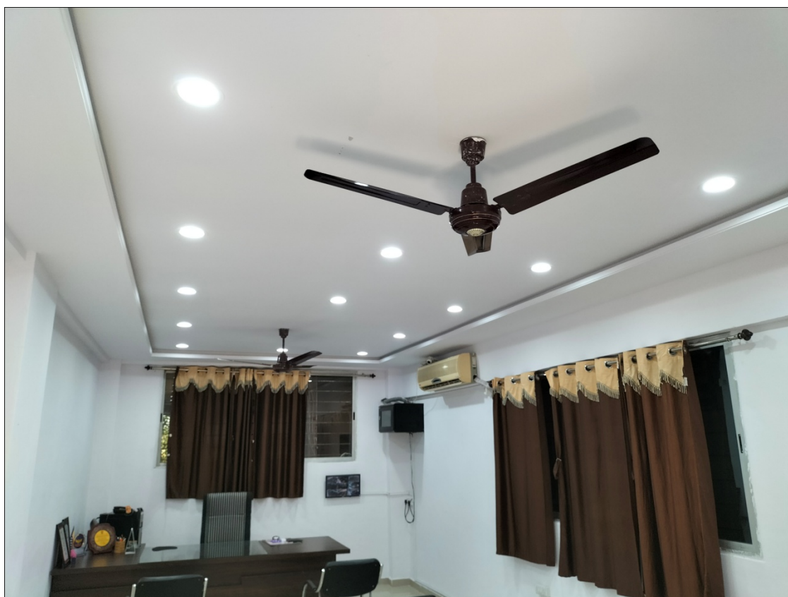
Concealed LED Lights fixed in Principal Cabin.
